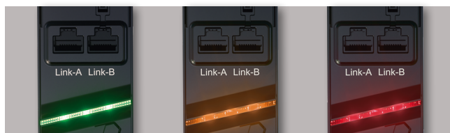
See alerts on the PDU for field technicians
